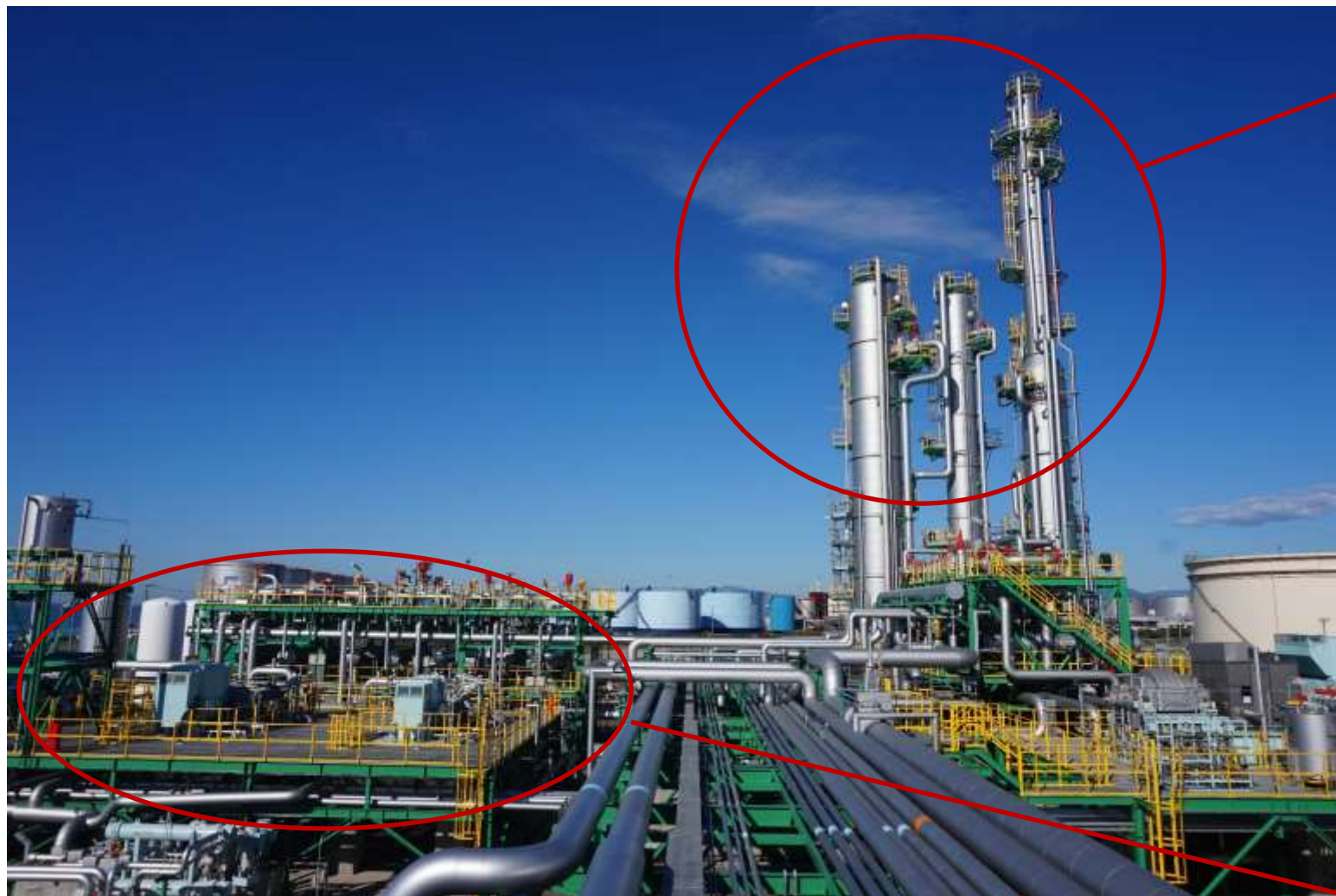
CO 2 Capture Facility
